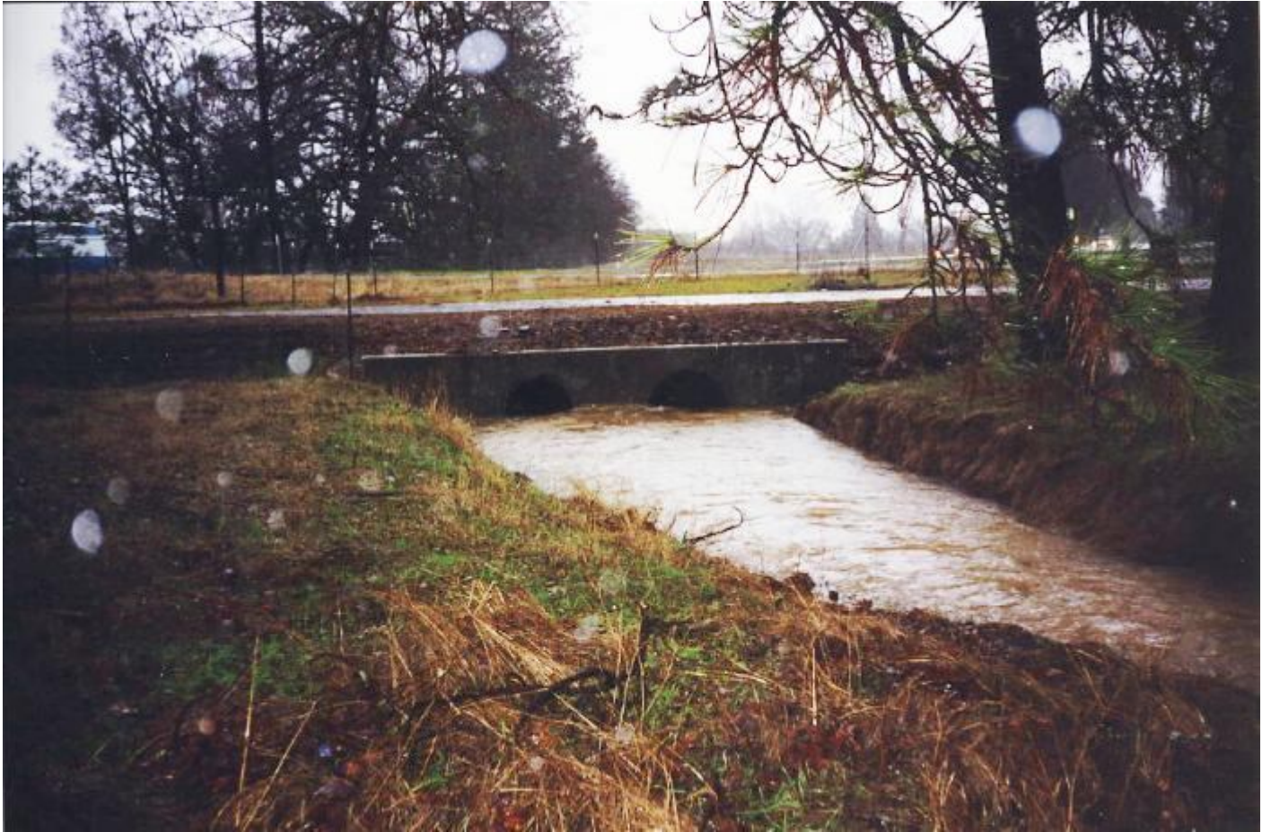
THE 3' AND 4' CULVERTS THAT WERE BLOCKED
